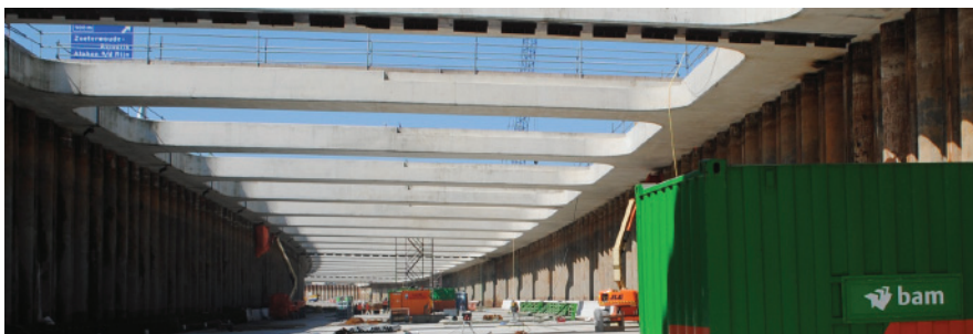
The A4 Burgerveen tunnel in Holland. Our panels ready to be installed.
